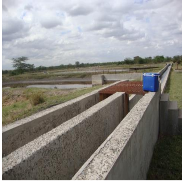
Ponds created for the safe disposal of effluent for a certain industry in Mavoko
