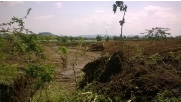
Gituamba dam: Before rehabilitation
