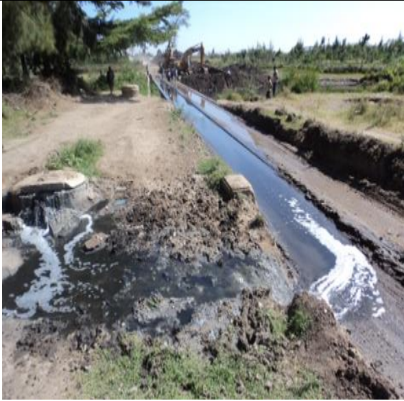
Perforated Manholes at Mavoko Sewer Line
